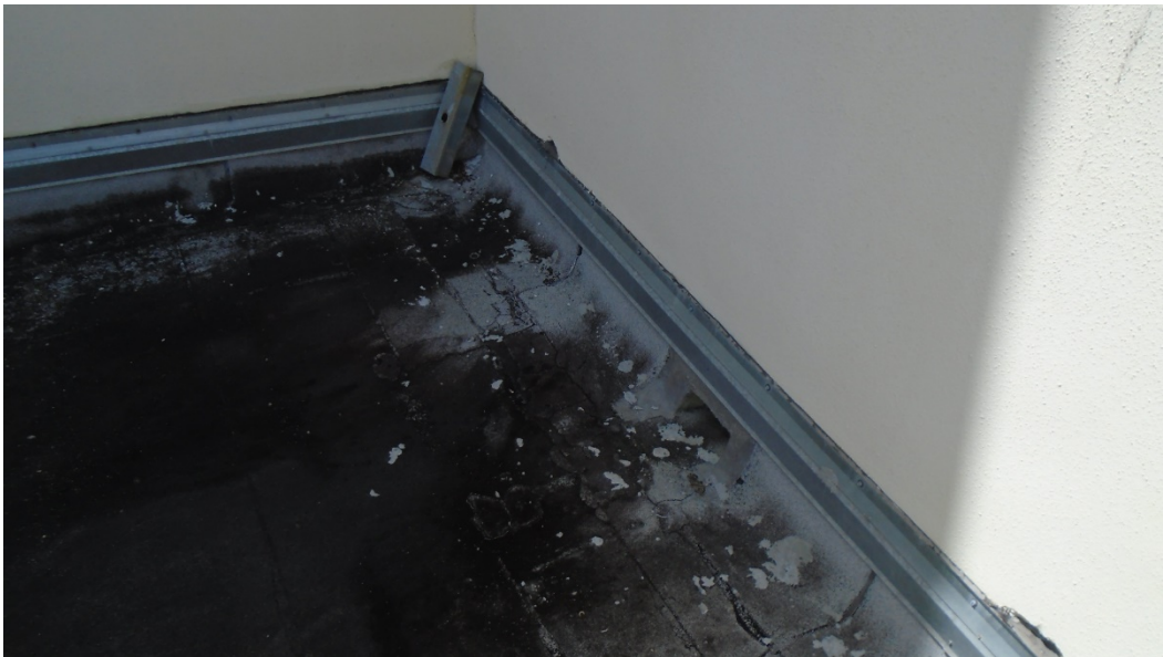
Photo 45: Low roof area 2 per Advance Roofing Report over entry at north side of building has damaged roofing exhibiting wear and deterioration. Roofing membrane has loss of granules.
