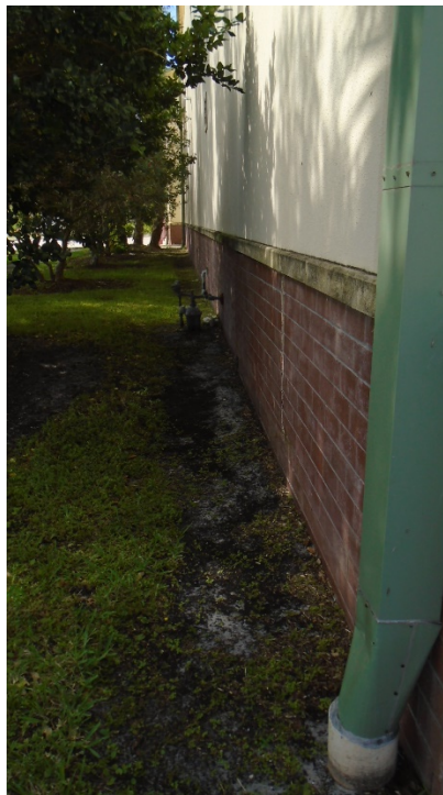
Photo 18: Rain water leaders at building perimeter drains to unknown underground areas.
