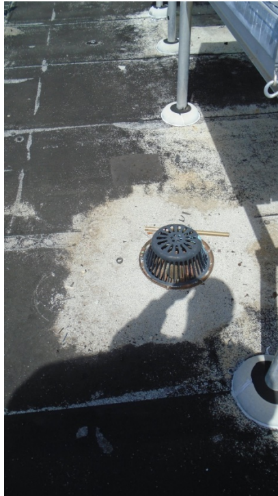
Photo 40: Loose granules from deteriorated roof membrane are accumulating around drains in roof area 3.
