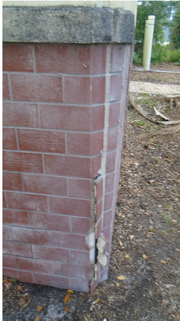
Photo 27: Damaged 4" split face brick veneer. South west building elevation.
