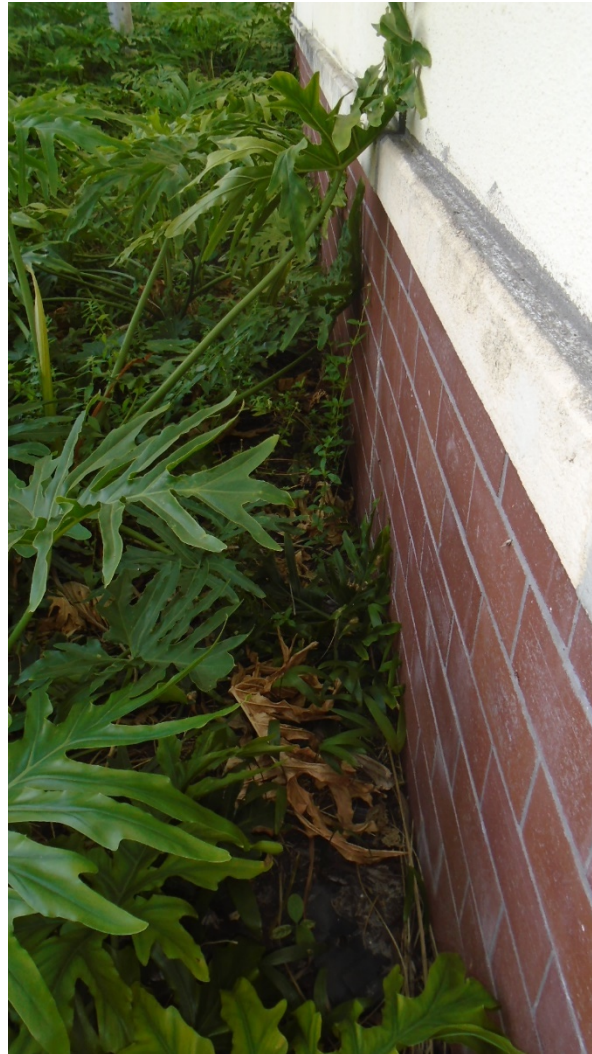
Photo 13: Landscaping area building west elevation. Landscaping built up against wall.
