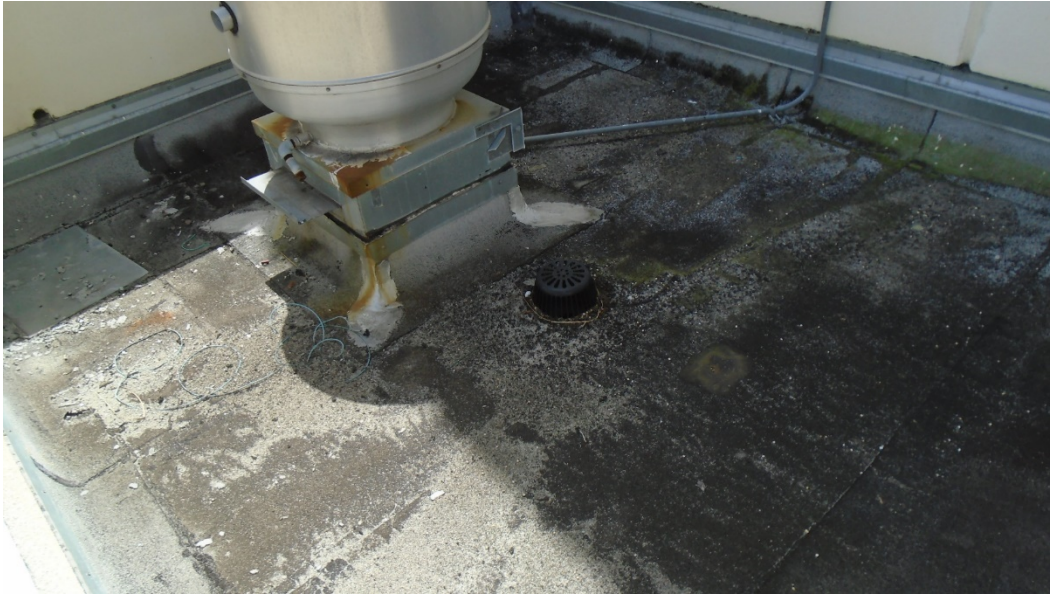
Photo 44: Low roof area 2 per Advance Roofing Report over entry at north side of building has damaged roofing exhibiting wear and deterioration. Roofing membrane has loss of granules.
