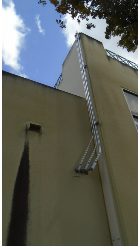
Photo 4: Faded paint on walls with mold and mildew stains. South building elevation.
