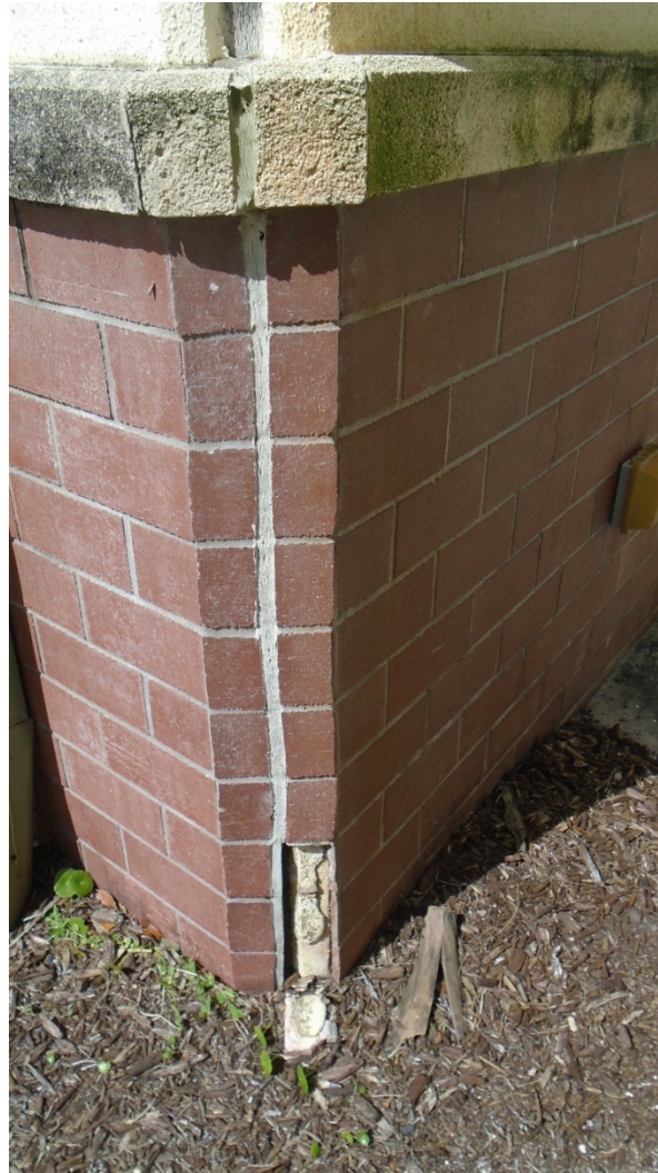
Photo 24: Damaged 4" split face brick veneer. East building elevation – fire truck storage.
