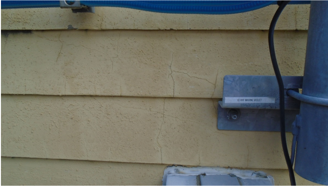
Photo 42: Cracks in wall to decorative finish adjacent to roof area 3 and over stair#2.
