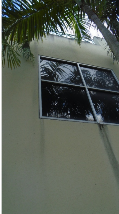
Photo 6: Faded paint on walls with mold and mildew stains. South building elevation.
