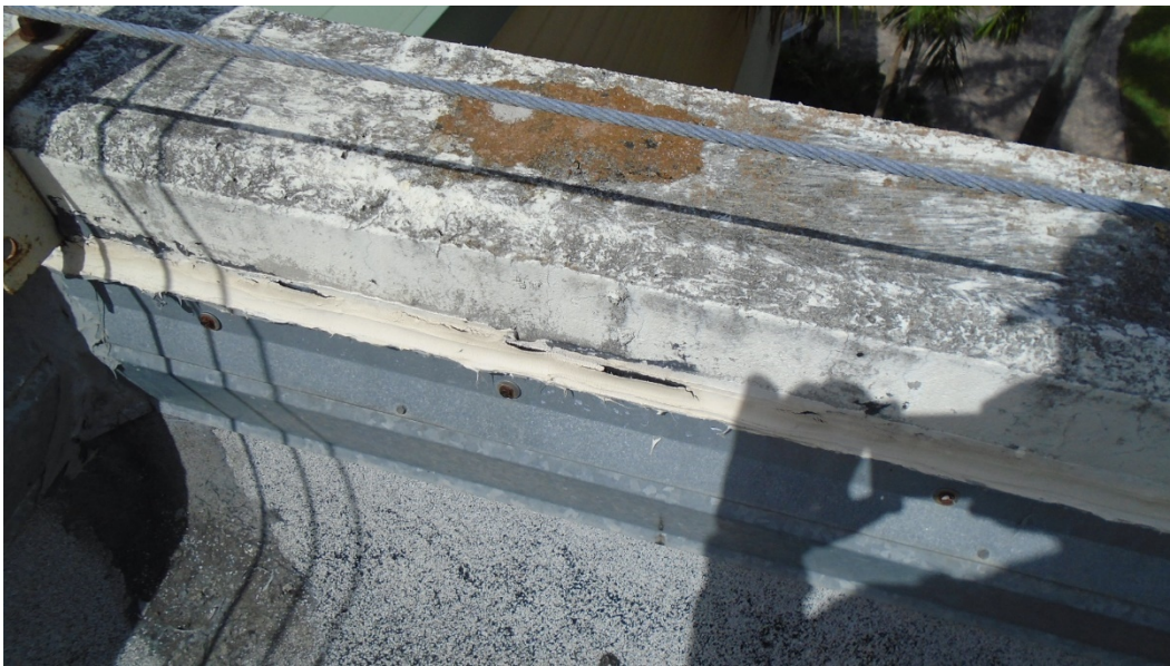
Photo 43: Failed sealant at flashing of roof area 3 located over stair#2.
