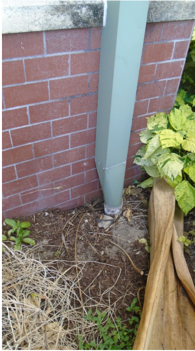
Photo 17: Rain water leaders at building perimeter drains to unknown underground areas.
