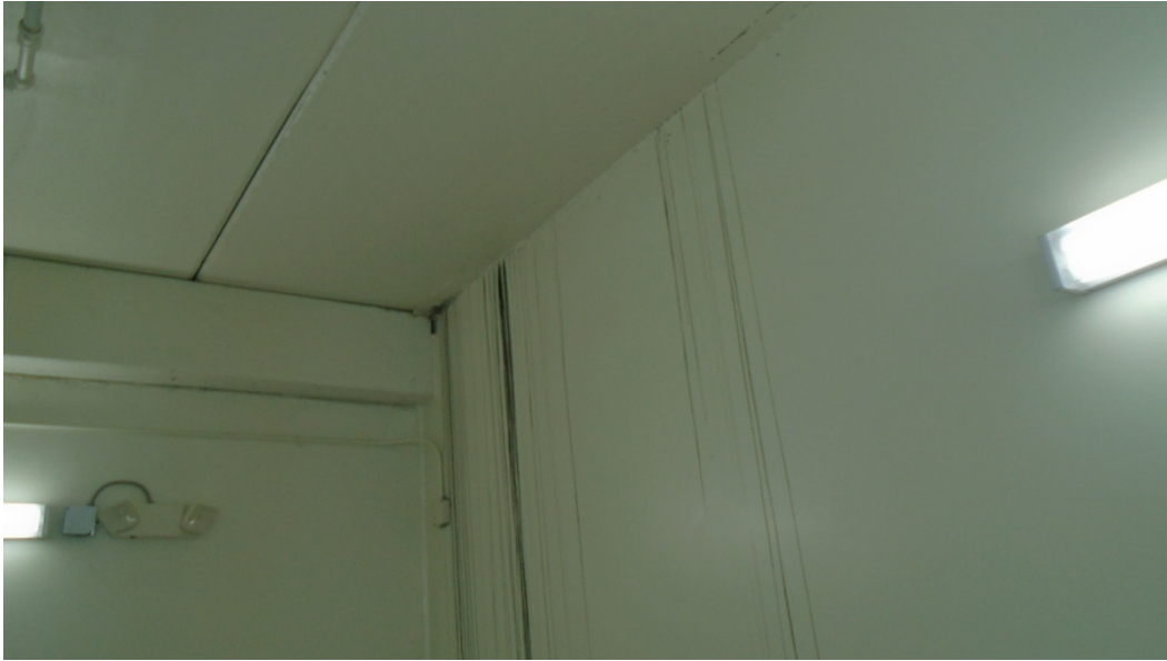
Photo 35: Water leaks stains inside stair#2.
