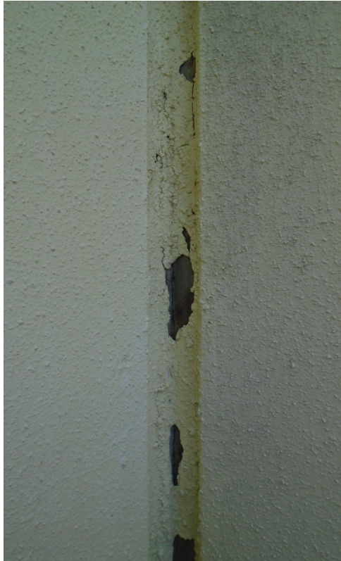
Photo 10: Failed paint over building concrete wall joint sealant.
