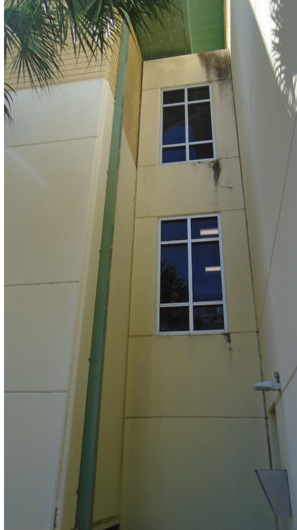
Photo 3: Faded paint on walls with mold and mildew stains. North building elevation.
