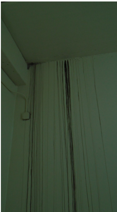
Photo 36: Water leaks stains inside stair#2.
