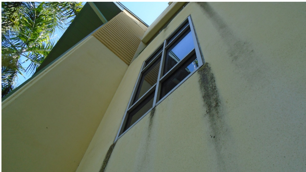
Photo 2: Faded paint on walls with mold and mildew stains. West building elevation.
