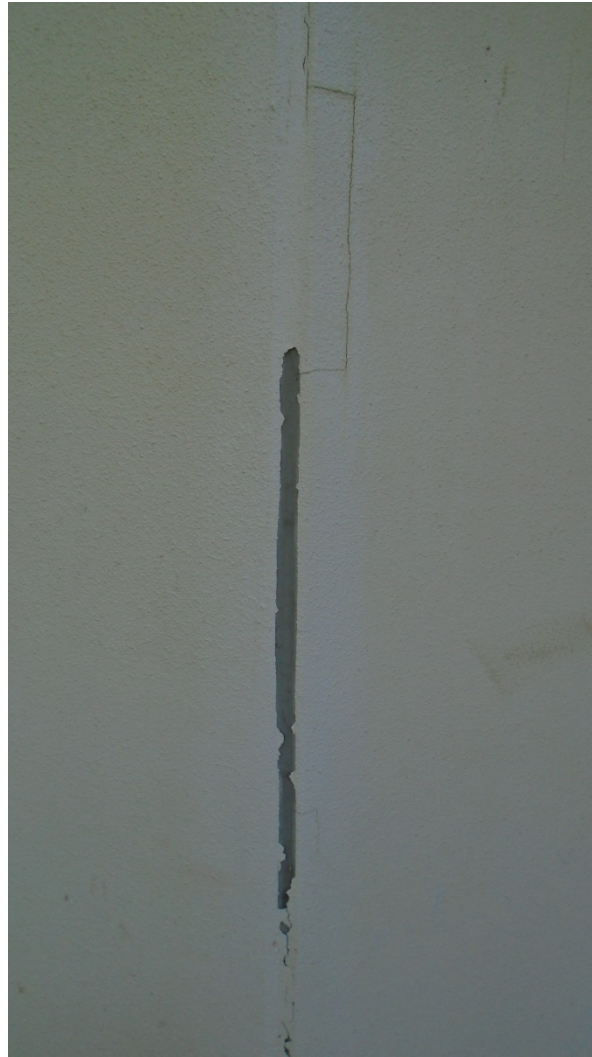
Photo 8: Failed paint over building concrete wall joint sealant.
