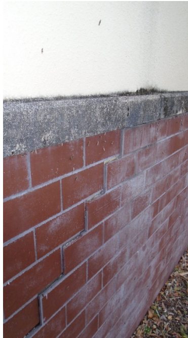
Photo 25: Damaged and loose 4" split face brick veneer. South building elevation.
