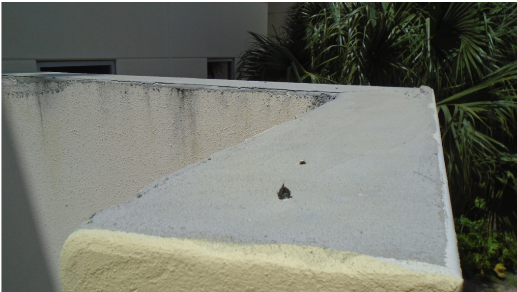
Photo 47: Low roof over entry area at north side of building has damaged stucco over top of parapet wall in roof area 2 per Advance Roofing Report. Stucco is cracked, spalled and loose.
