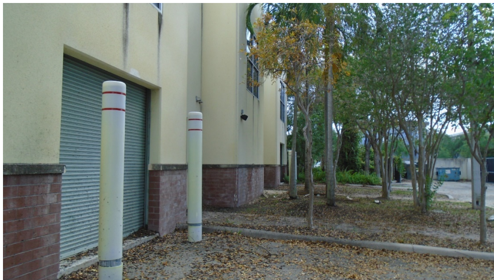
Photo 5: Faded paint on walls with mold and mildew stains. South building elevation.
