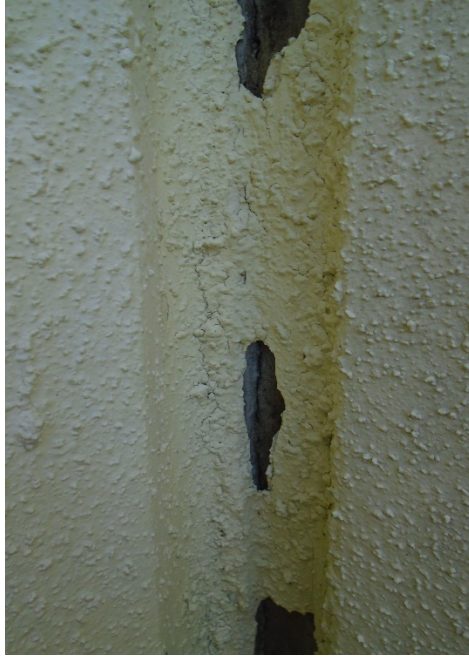
Photo 9: Failed paint over building concrete wall joint sealant.
