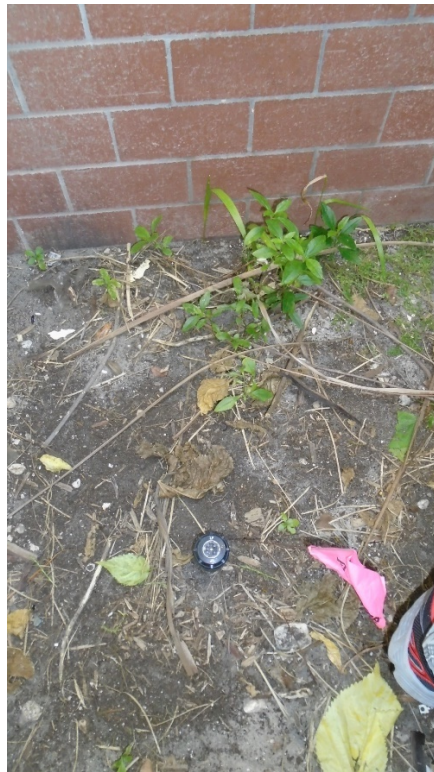
Photo 15: Irrigation system within landscaping area and near building walls.
