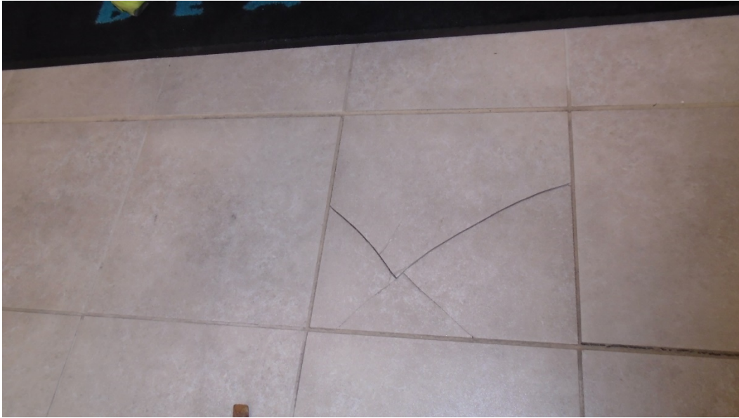
Photo 31: Crack tile in vestibule interior at interface between building area at grid 5.
