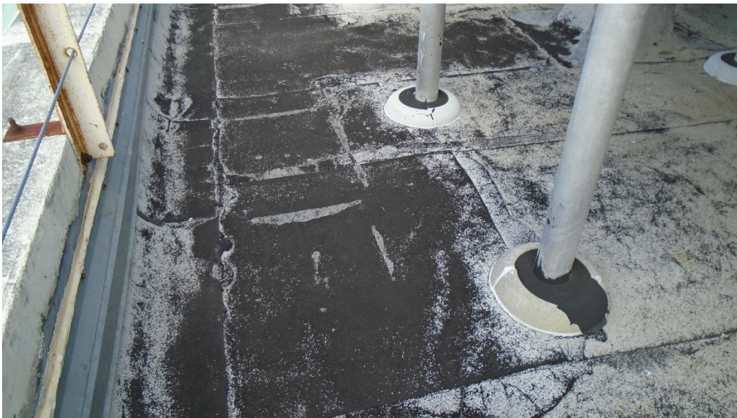
Photo 41: Loss of granules from deteriorated roof membrane in roof area 3. Excessive wear of membrane.
