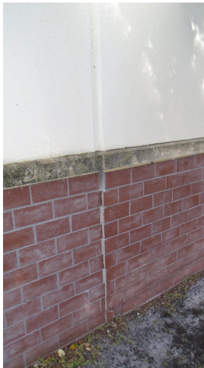
Photo 23: Damaged and de-bonded 4" split face brick veneer. East building elevation.
