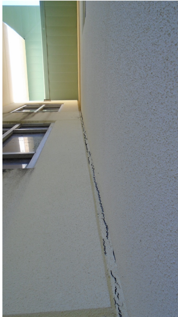
Photo 28: Failed sealant at interface between building area grid 5 front entrance vestibule south elevation.
