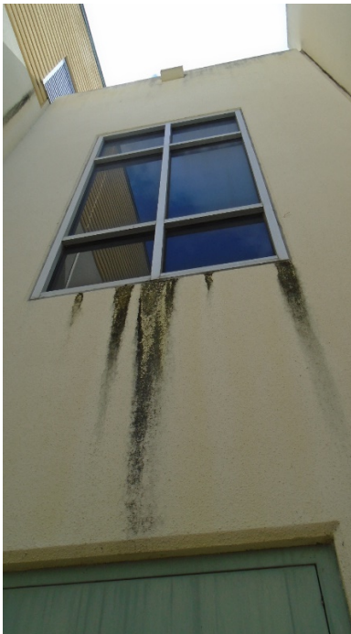
Photo 7: Faded paint on walls with mold and mildew stains. West building elevation.
