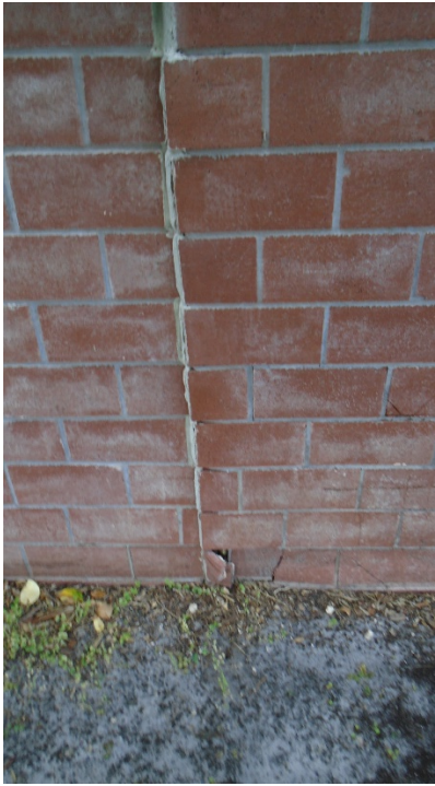
Photo 22: Damaged and de-bonded 4" split face brick veneer. East building elevation.
