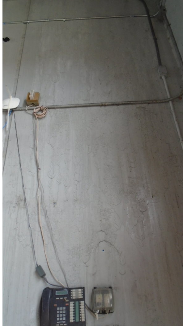
Photo 37: Damaged paint on wall adjacent to stair#2 inside fire truck storage.
