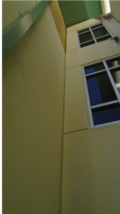
Photo 29: Failed sealant at interface between building area grid 5 front entrance vestibule north elevation.
