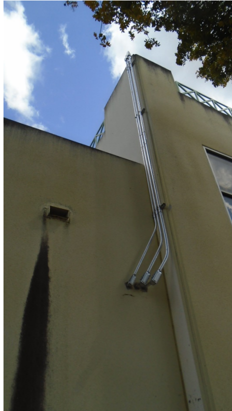
Photo 4: Faded paint on walls with mold and mildew stains. South building elevation.
