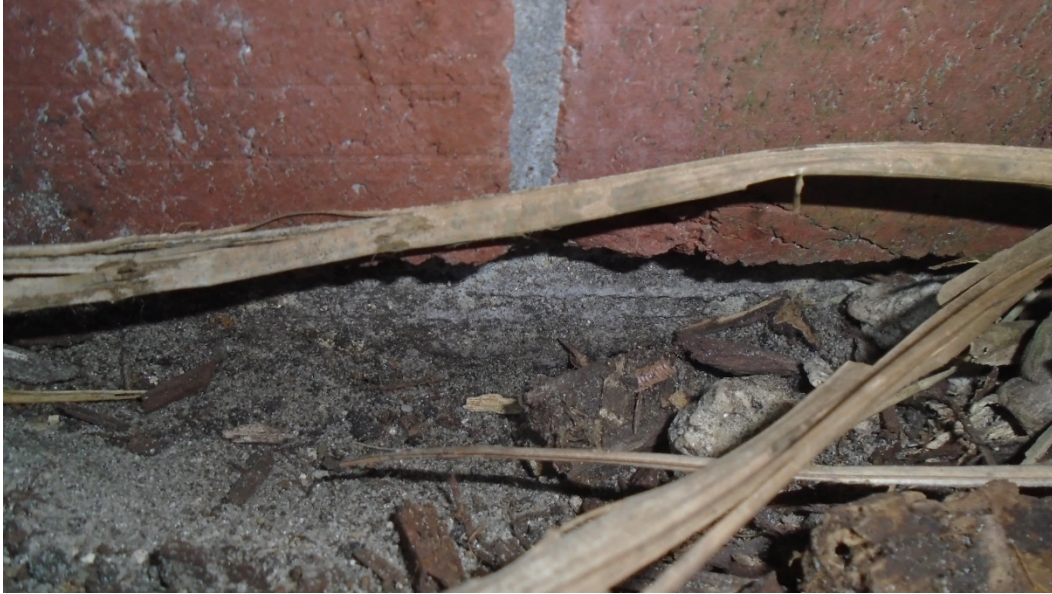
Photo 20: Close view of bottom portion of decorative 4" split face brick veneer found throughout building with existing bare concrete wall behind. No waterproofing on existing concrete wall.
