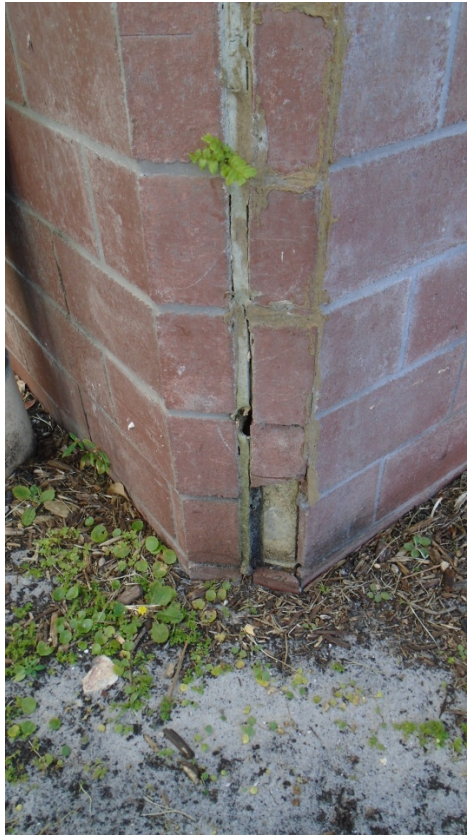
Photo 21: Damaged 4" split face brick veneer. North east building elevation.
