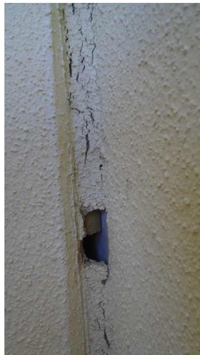
Photo 30: Failed sealant at interface between building area grid 5 front entrance vestibule south elevation.
