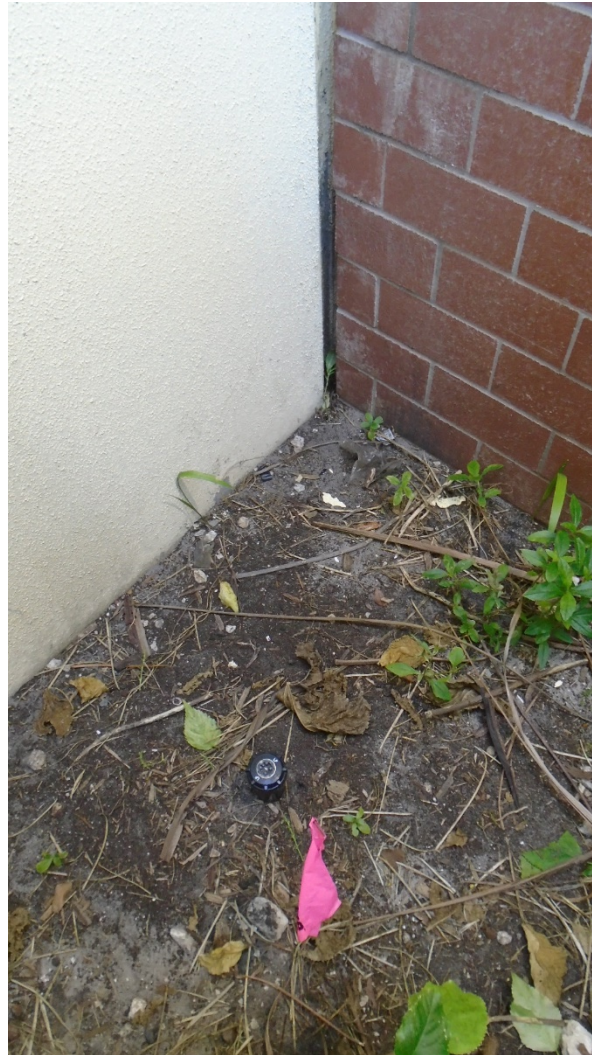
Photo 16: Irrigation system within landscaping area and near building walls.
