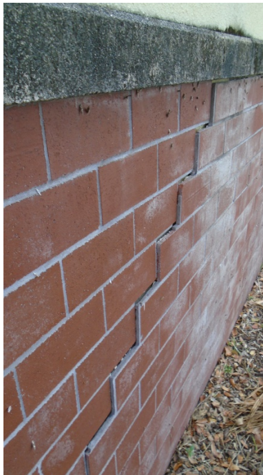
Photo 26: Damaged and loose 4" split face brick veneer. South building area.
