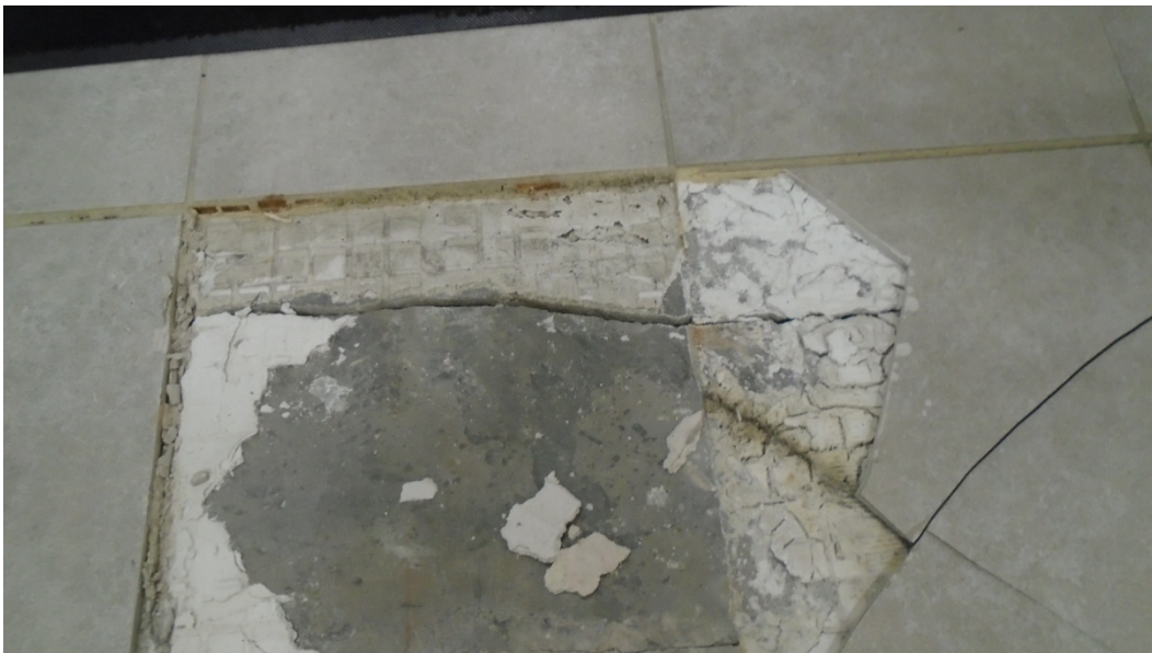
Photo 32: Tile removed interior exposing fracture in topping slab over structural hollow core plank floor system. Damage is located at 2 nd & 3 rd floors in vestibule at interface between building areas at grid 5.
