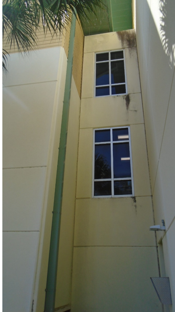
Photo 3: Faded paint on walls with mold and mildew stains. North building elevation.
