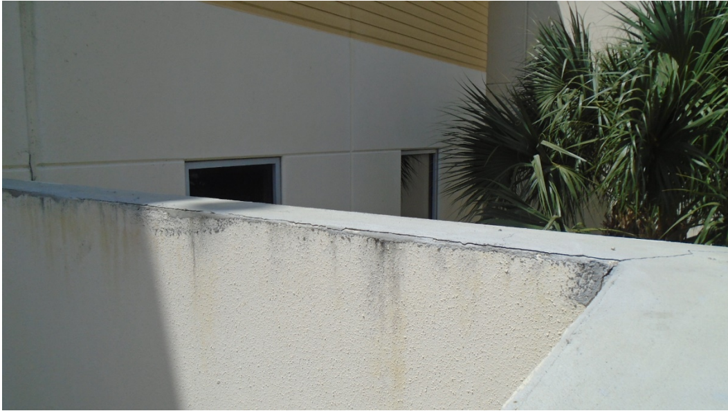
Photo 46: Low roof over entry area at north side of building has damaged stucco over top of parapet wall in roof area 2 per Advance Roofing Report. Stucco is cracked, spalled and loose.
