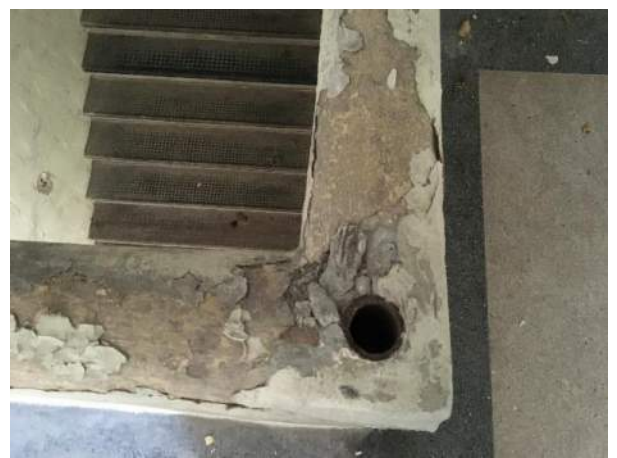
South Stair – Railing Removed at top of railing
