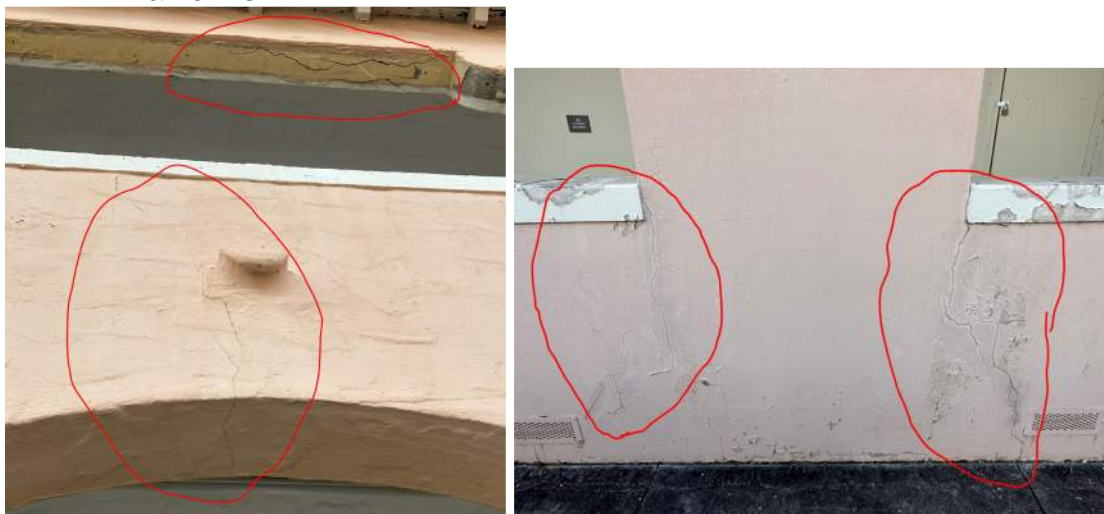
Photos 29 & 30 – Cracks in various portion of west side wall of north wing
