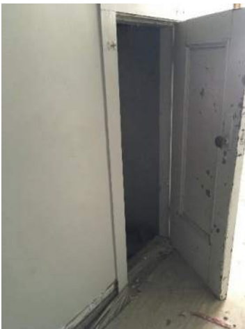
Room 121D – Existing door not in compliance
