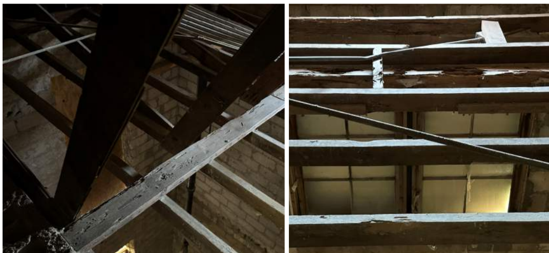
Photos 7 & 8 – Termite damage in the wood framing above the restrooms.
