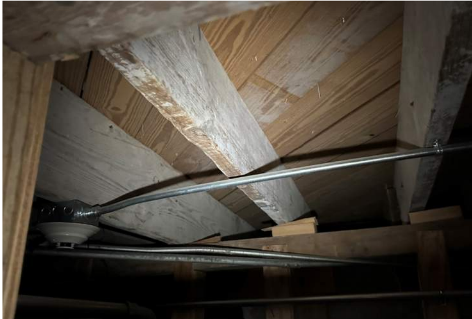
Photo 18 – Another location with multiple shims under the floor joists
