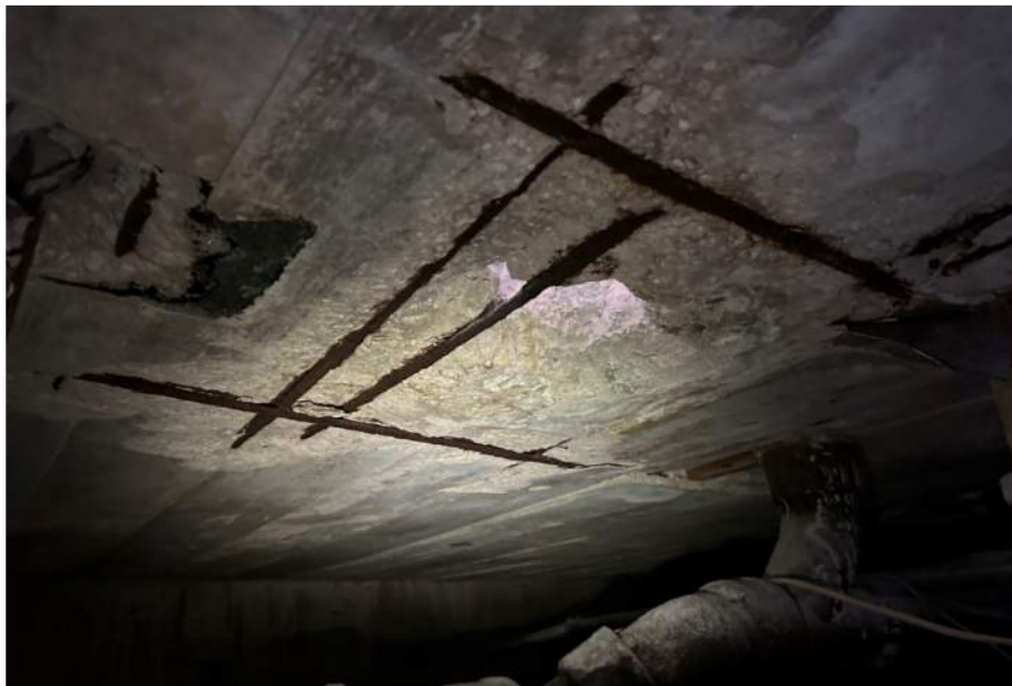
Photo 38 – Exposed rebars with severe rusting in the north wing restroom slab
