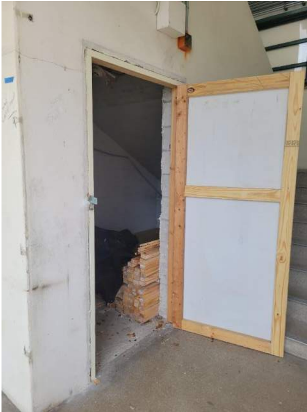
Room 115 – Room under stair to be sealed as it is not in compliance
