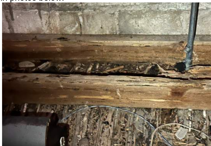
Photo 9 – Severe termite damage in ceiling framing
