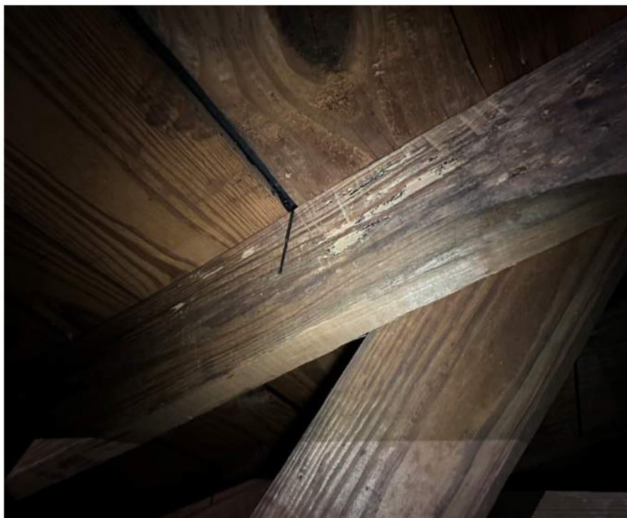
Photo 6 – Roof Framing with termite damage
