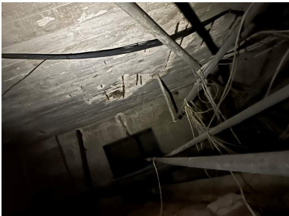
Photo 39 – Exposed and rusted rebar on the slab below the stairwell.
