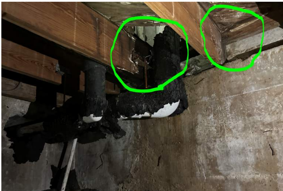
Photo 23 – Damaged floor joists at A/C pipes.
