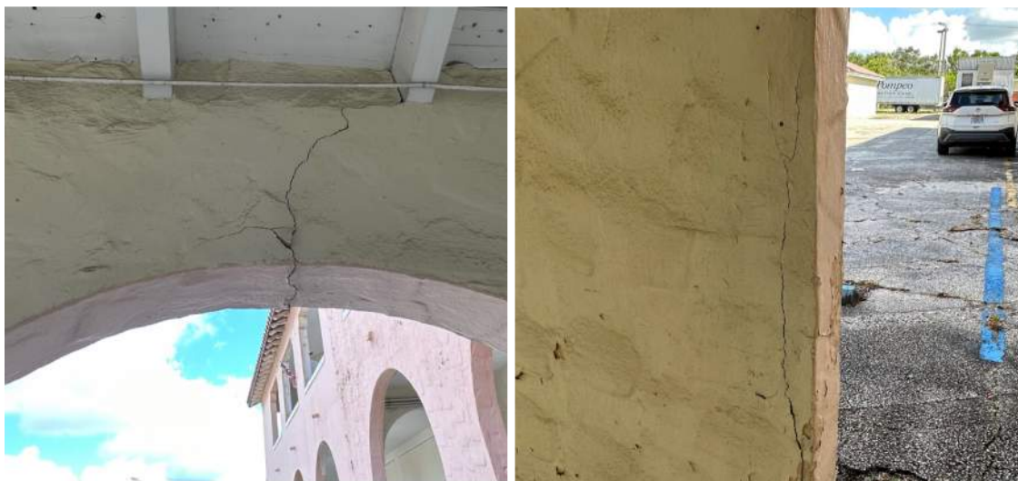
Photos 27 & 28 – Cracks in the concrete arch on the north side of auditorium
