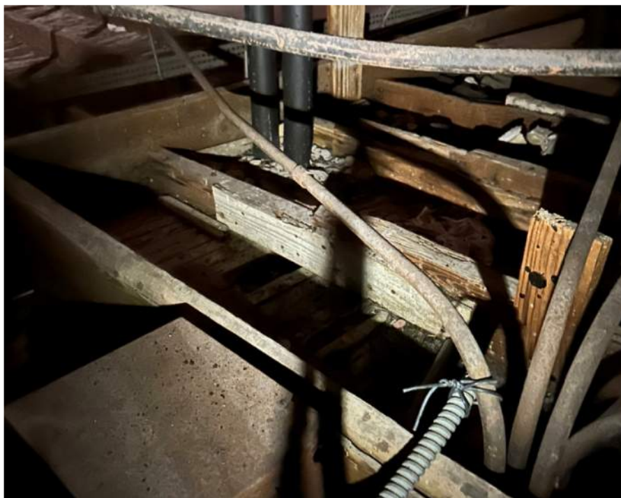
Photo 5 – Shows ceiling framing with splices, cuts or other damages
