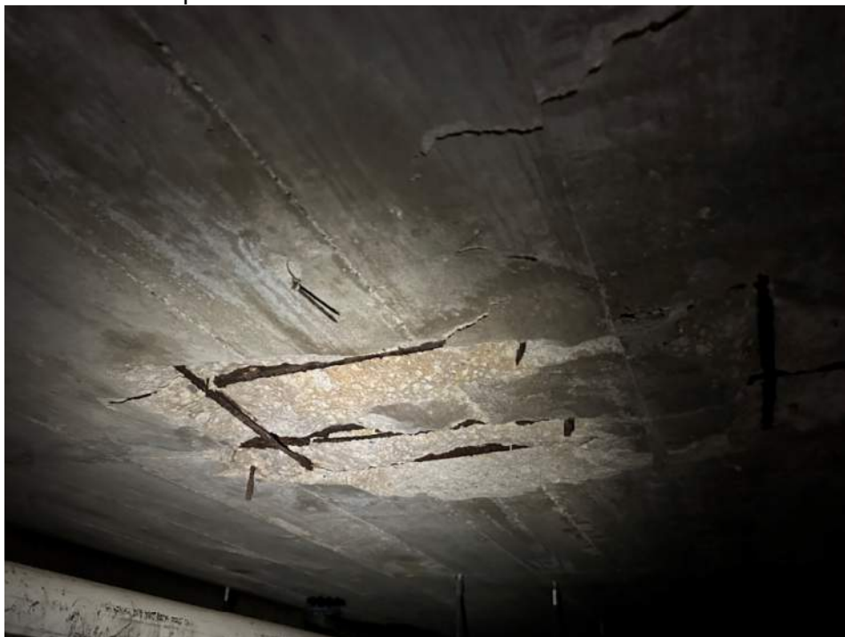
Photo 40 – Bottom of corridor slab with spalling and exposed rusted rebar
