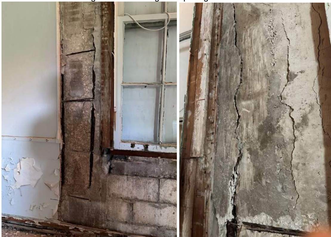
Photos 35 & 36 – Another classroom wall with cracking and spalling tie column
