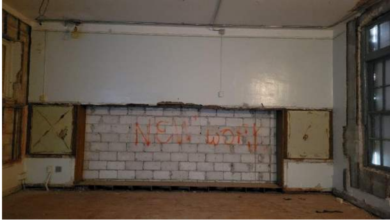
Room 112 – Void Left by casework in North Wall
