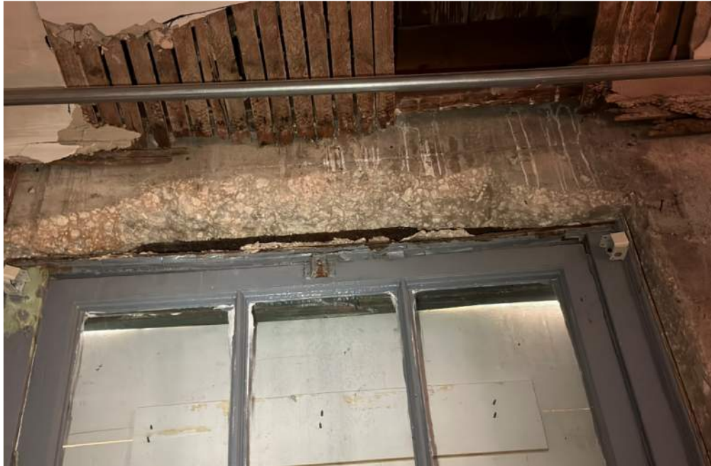
Photo 37 – Spalling with rusted rebar in the lintel in one of the classrooms
