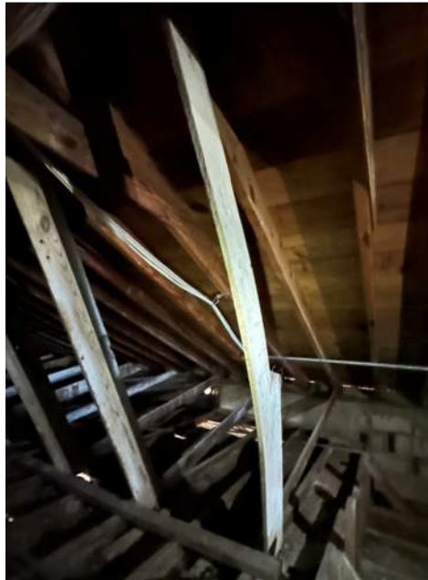
Photo 13 – One of the truss diagonals with cut and reduced section is bowing.
