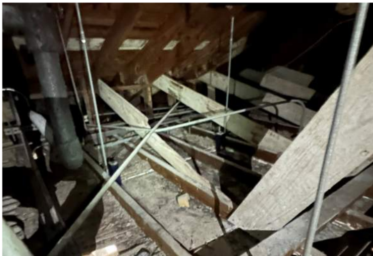
Photo 14 – Another diagonal 1x6 with cut at an electrical conduit.
