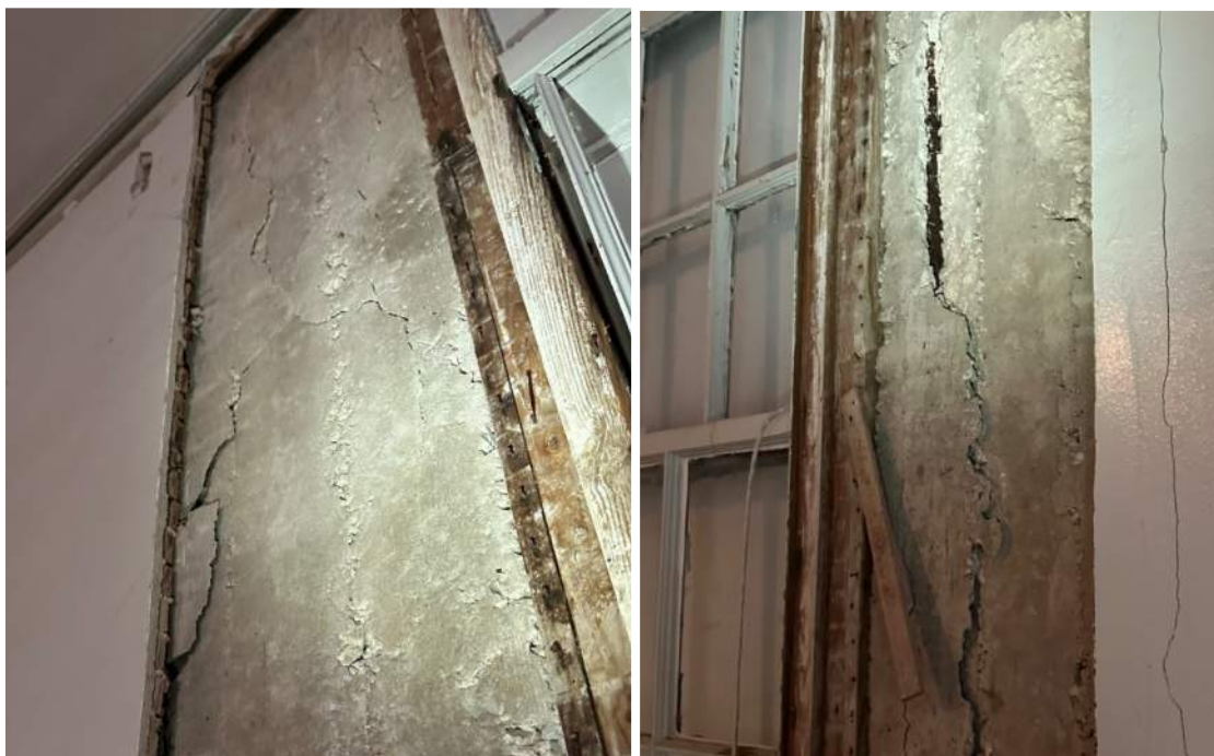
Photos 33 & 34 showing severe cracking and spalling in tie columns in classroom wall
