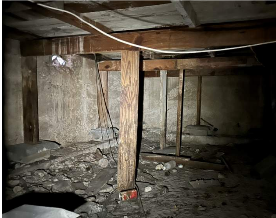
Photo 22 – Floor framing supported by wood posts and no foundations
