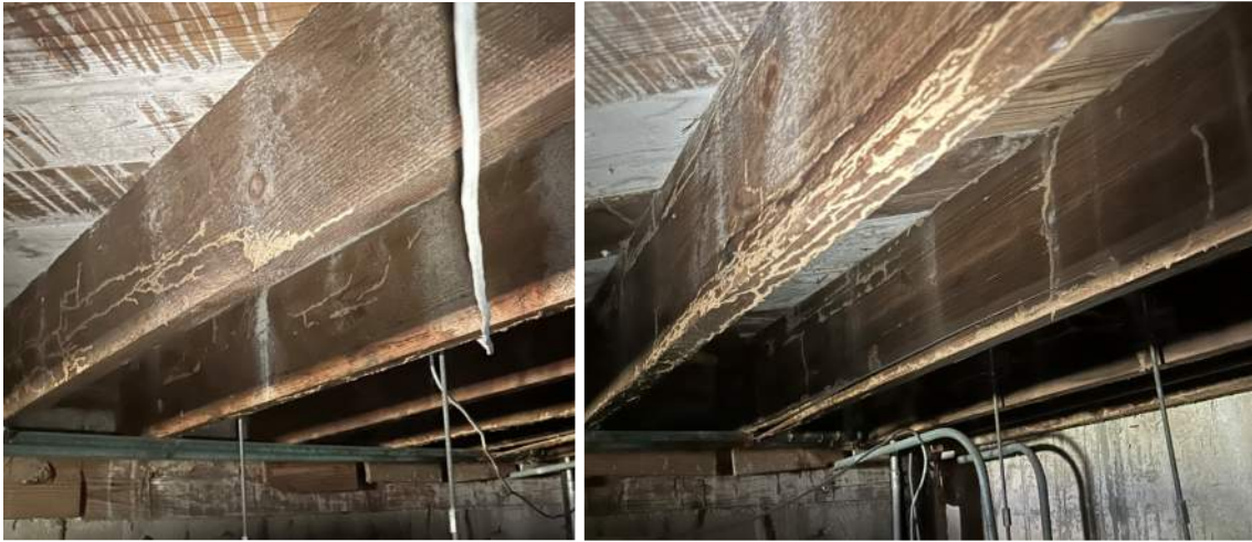
Photos 24 and 25 shows extensive termite damage to the floor framing under Room 112
