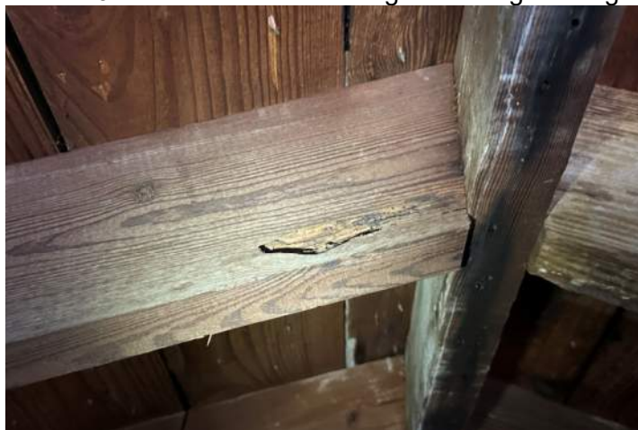
Photo 10 – Termite damage in the roof framing
