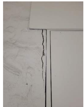
Rm. 103 – Cracks in wall at door
