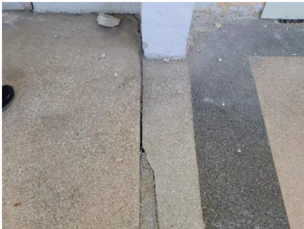
Exterior Flooring Condition – 2 nd Floor Outdoor corridor outside of Room 127
