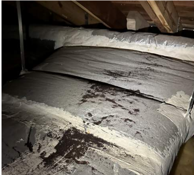
Photo 3 – Termite dust below the roof deck areas with termite damage
