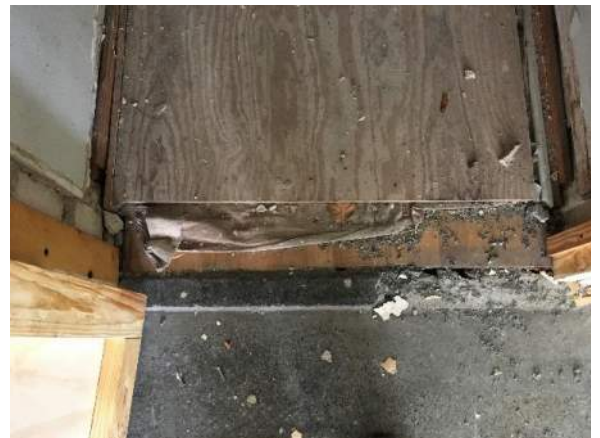
Room 120 – Existing threshold damaged at entrance
