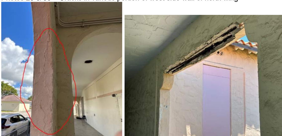
Photos 31 & 32 showing more cracks and spalling in exterior concrete walls
