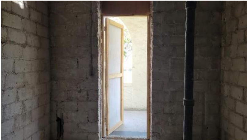
Room 111 – RWL location off North wall to be addressed
