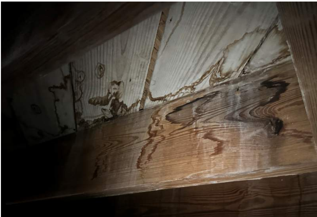
Photo 21 – Stain from water leaks and some wood rotting (darker spots)
