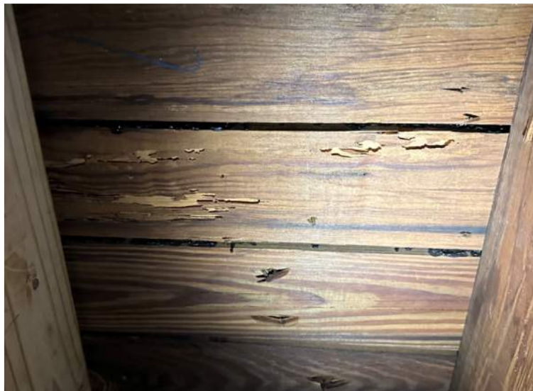
Photo 2 – Termite damage in roof decking
