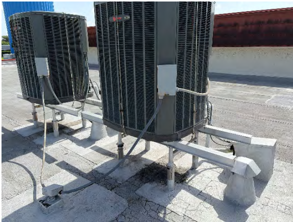
Typical AC unit with air conditioning stand
