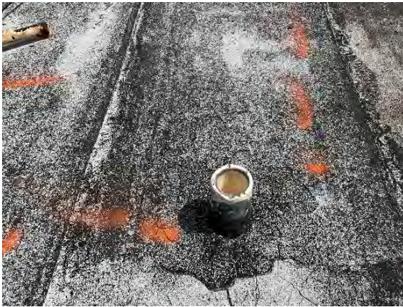
Typical plumber vent
