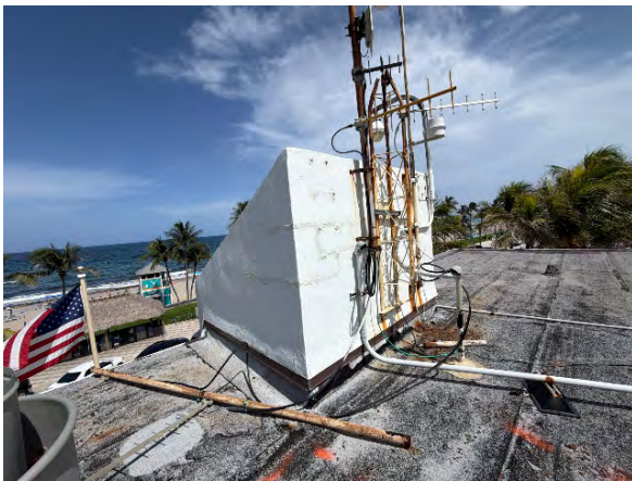
Typical mansard with satellite equipment Observation all rusted out
