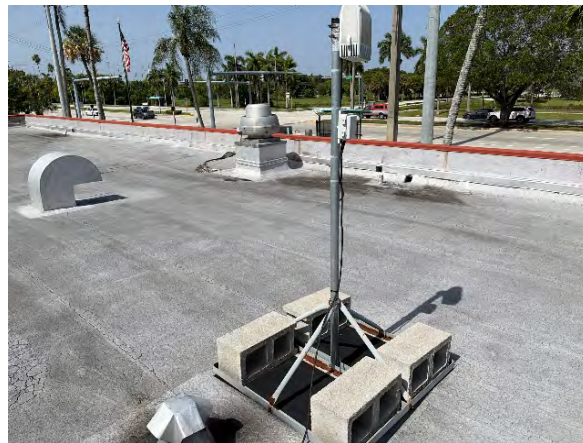
Typical antenna with concrete blocks mounted
