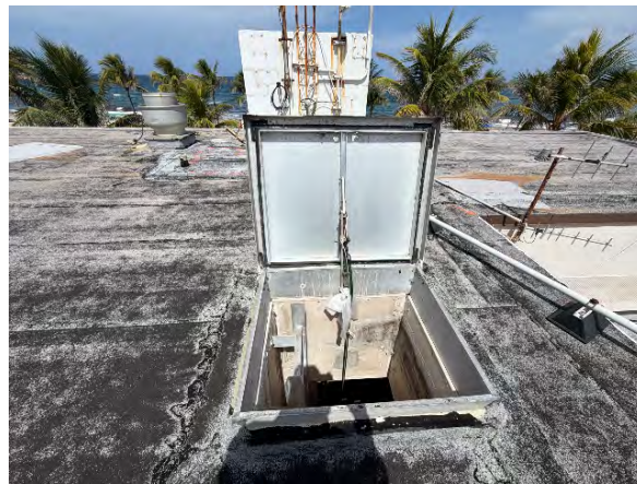
Typical roof hatch
