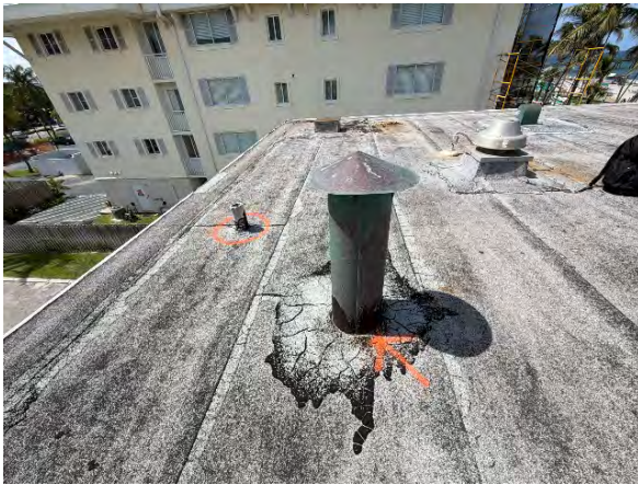
Typical APV vent
