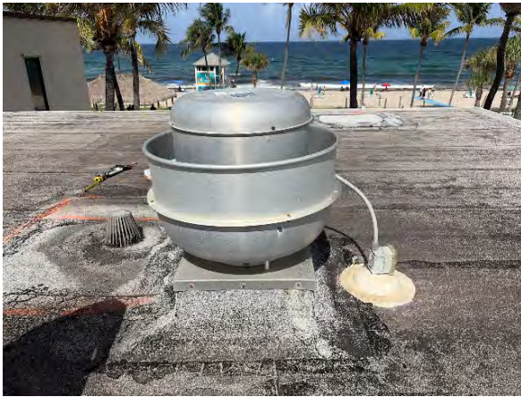
Typical exhaust fan with electrical conduit, flashing detail
