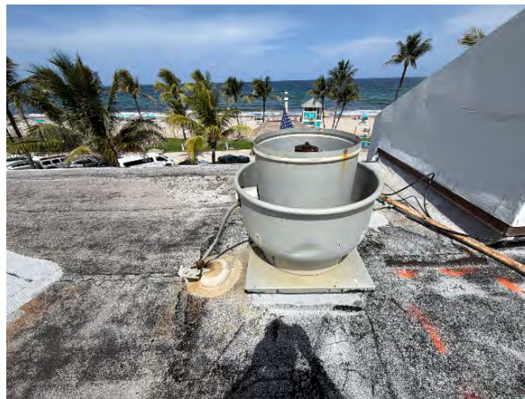
Typical exhaust fans Observation abandoned, exposed electrical wire
