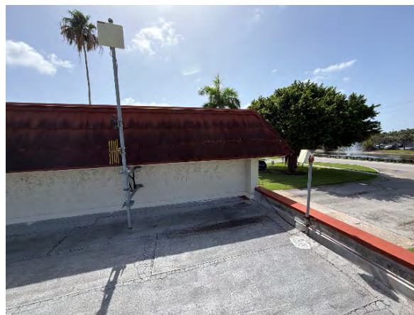
Typical antenna mounted over wall
