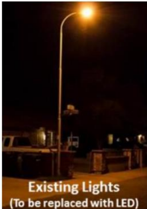
Existing 2200 Kelvin HPS
